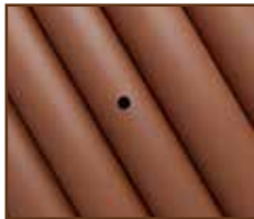
Small external outlet hole
